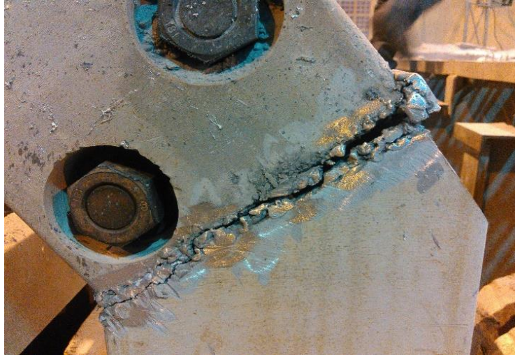
Figure 3. Example of weld damage resulting from initial poor quality
